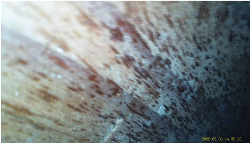
4074 #5: Stained plywood moisture
