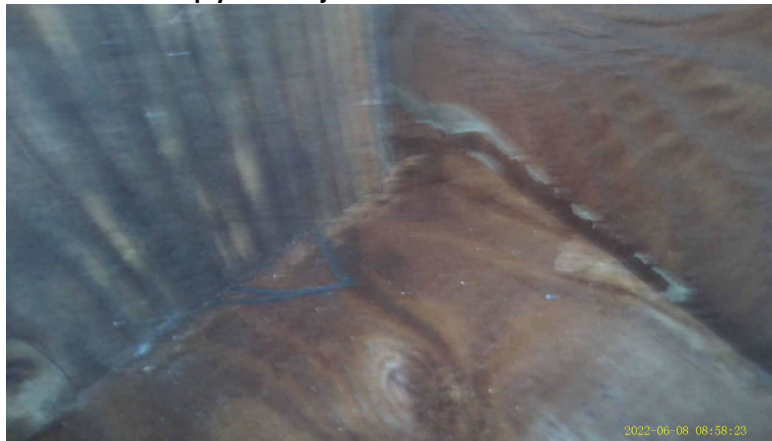
4062#4: Stained plywood & joist
