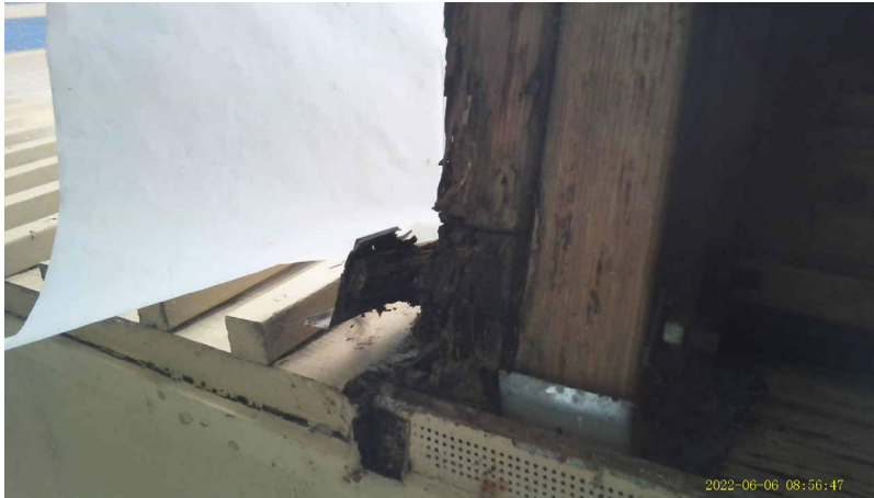
4074 #1: Trim moisture rot
