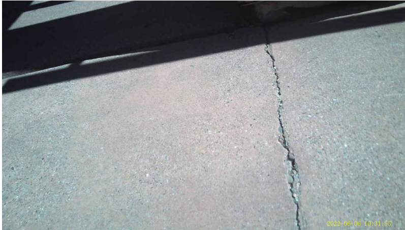
4074 #4: Concrete cracking tracking stained plywood moisture
