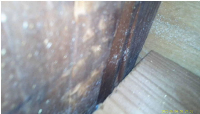
4062#7: Stained plywood & joist
