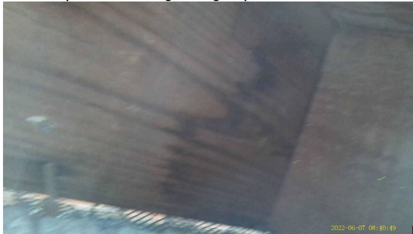
4086#3: Water stained moist member
