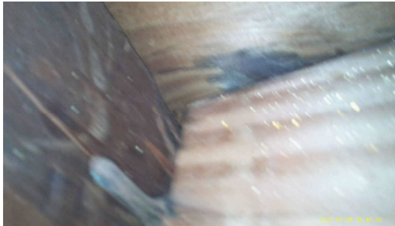
4062#2: Stained plywood & joist
