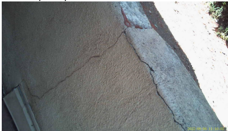
4074#7: Wall top cap stucco spalling
