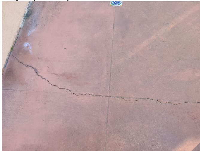
Bridgeway Concrete Deck Cracking
