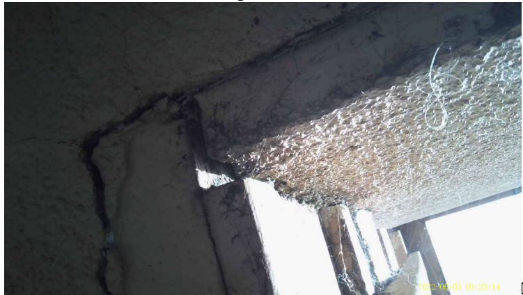
4050 #3: Deck Flashing Failure Dryrot
