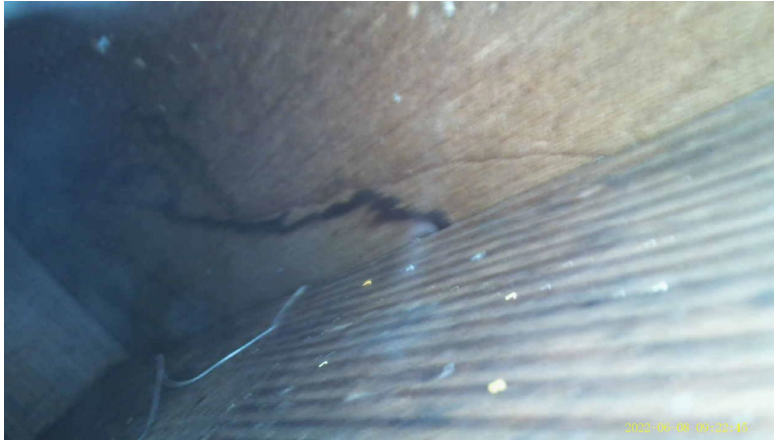
4062#5: Stained plywood & joist
