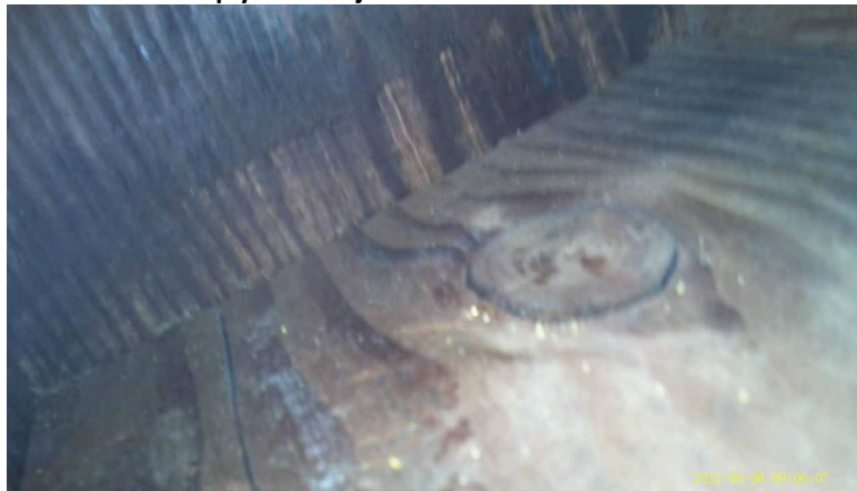
4062#3: Stained plywood & joist
