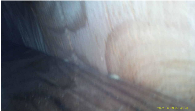
4062#6: Stained plywood & joist
