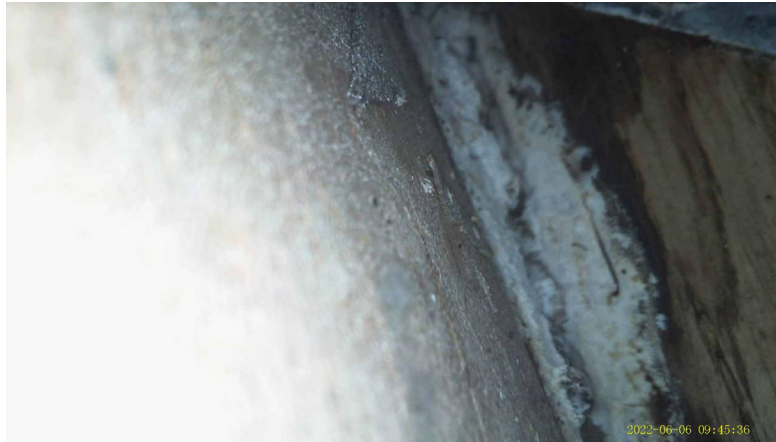
4072 #3: Dryrot within Joist Bay
